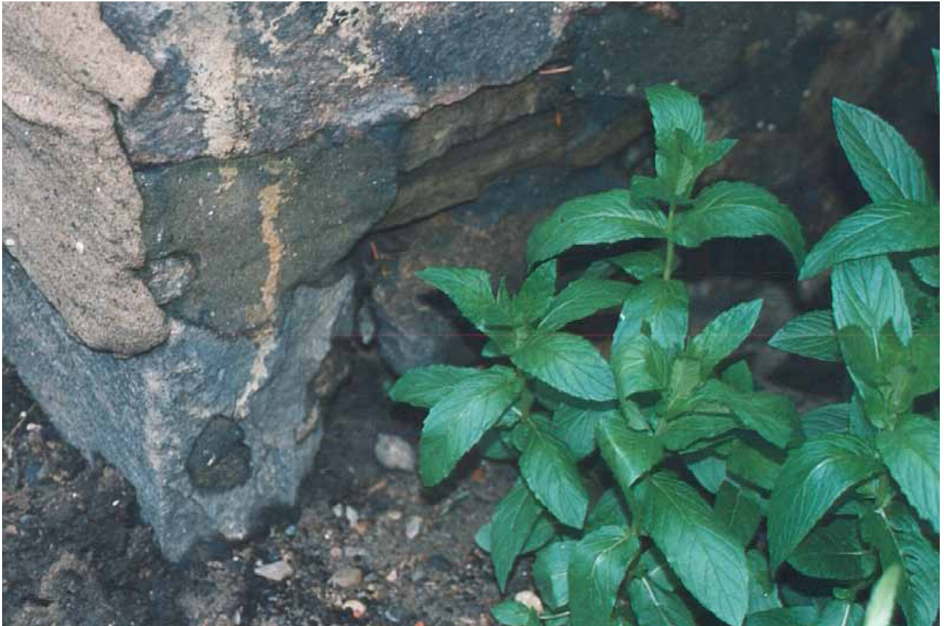
Figure 2. Water can enter the foundation wall above- and below-grade through deteriorated joints.
